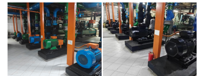
Before and after the circulating water pump retrofits
