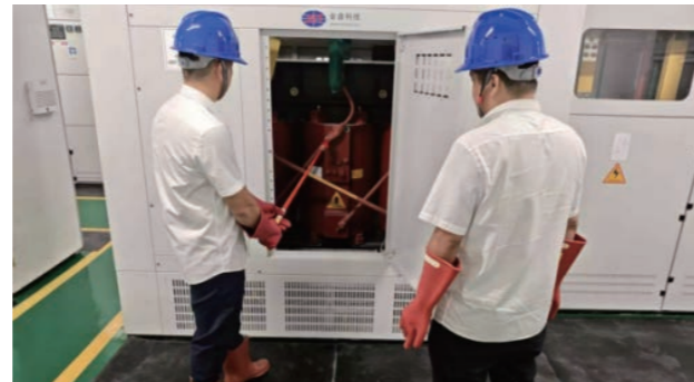
^ Adjusting the operations mode of transformers
