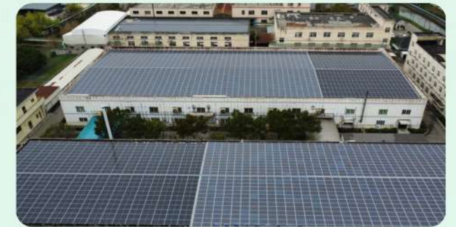
Our 1,118KW Rooftop Photovoltaic Project
