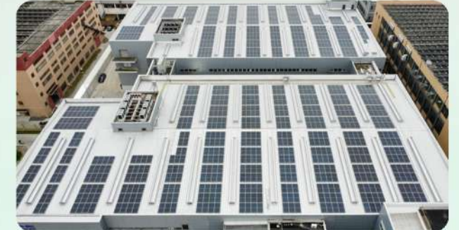
New Factory 650KW Rooftop Photovoltaic Project
