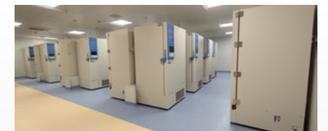
On-site delivery of the DW-HL860 Ultra-Low Temperature Freezers
