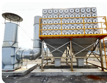
Welding Exhaust Gas Treatment Facilities (Newly-added)
