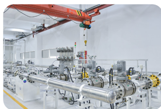
High-Pressure Loop Test Facility
