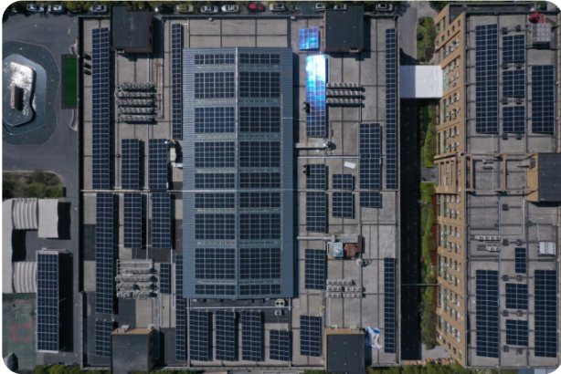
Hangzhou Photovoltaic Project
