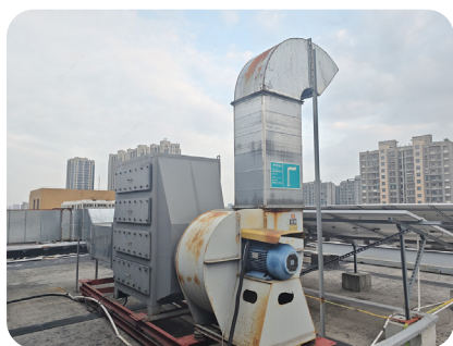
Fume Treatment System (Original)
