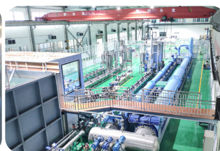
Large-Scale Water Loop Test Facility
