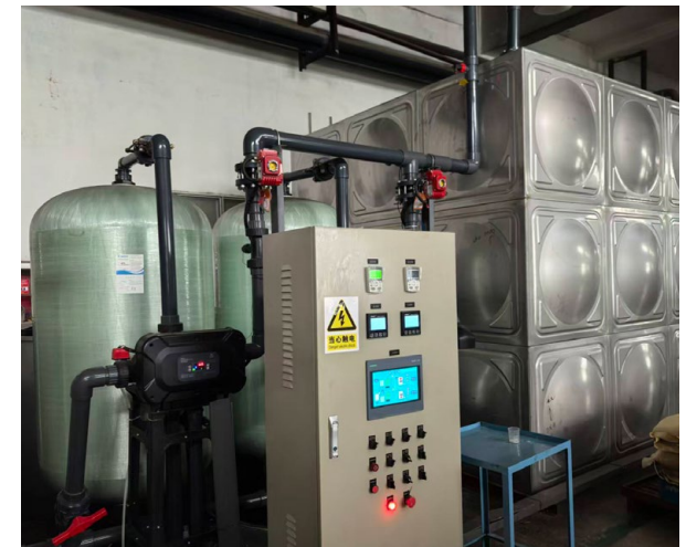
Dongying Factory Water Softening Ion Exchange System
