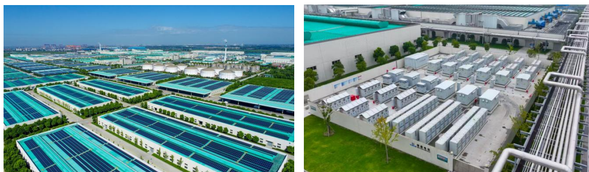
Hengli (Nantong) Industrial Park Photovoltaic Power Generation Project and Hengli (Nantong) Industrial Park Energy Storage Project
