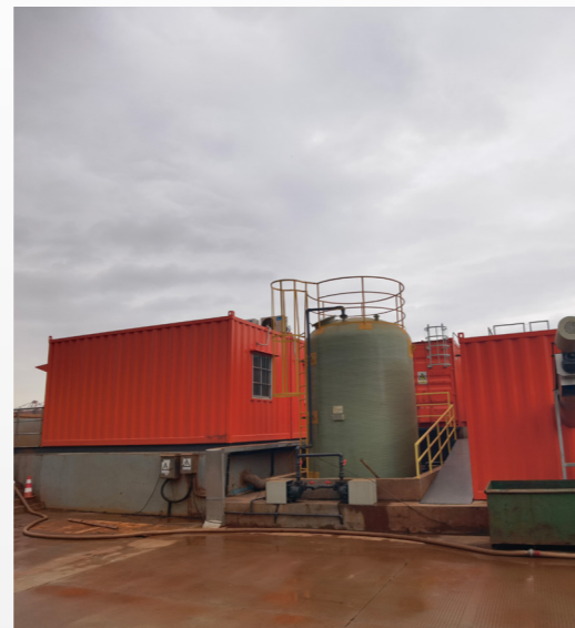
Sewage Treatment System of Beilun Ore Terminal Branch
