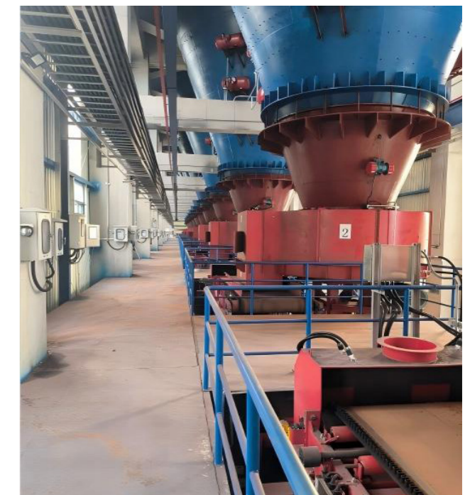
Nanjing Mingzhou Terminal Integrated Ore and Coal Processing Services
