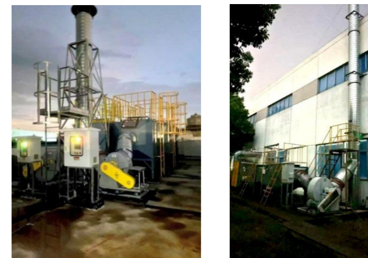
▲和林微纳普陀山路厂区废气设施
